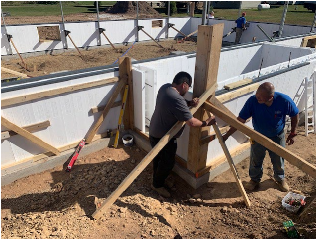
Melvin and Mark are setting concrete forms for the foundation to be poured.
